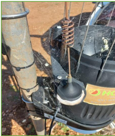
Rusted Antenna, resulting in bad signal connectivity. Inform iLeaf if any parts are rusted. This needs to be replaced
