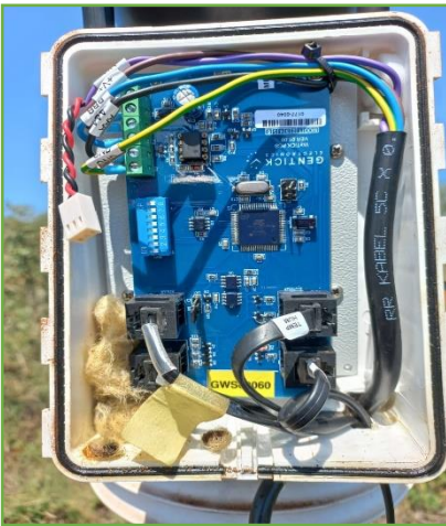
Spider webs, Gecko eggs and dust. Cause malfunctioning motherboard parts. Resulting in expensive logger replacement
