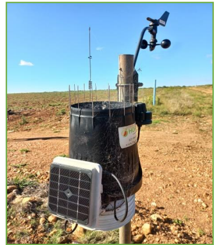
Station covered in spider webs or dust, means there is a high chance of more critters inside. Station needs a clean.
